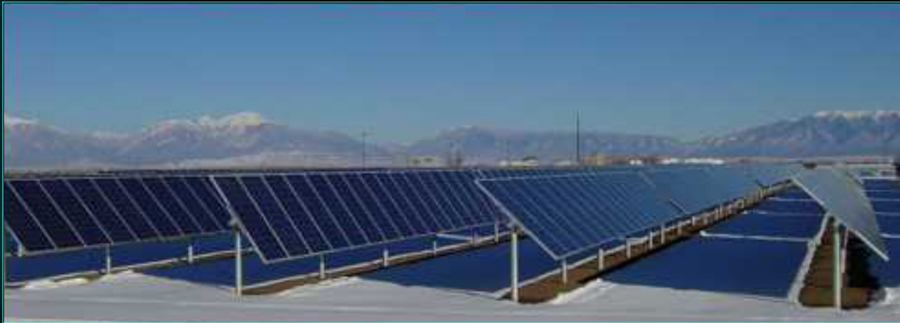
Alamosa Colorado 8.2 MW photovoltaic plant
